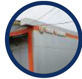
Cold Storage KKP cold storage
