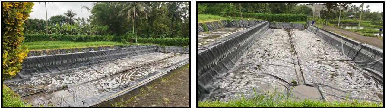
Gambar 42. Kolam HDPE (High Density Polyethylene)
